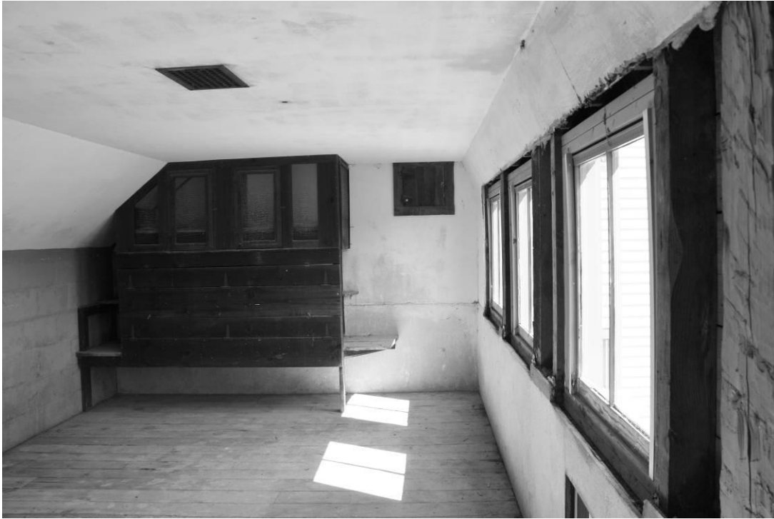
Photo # __16__ Description: Poultry barn, second floor interior (south building) Digital file name: NHA0010_16 Direction: north
