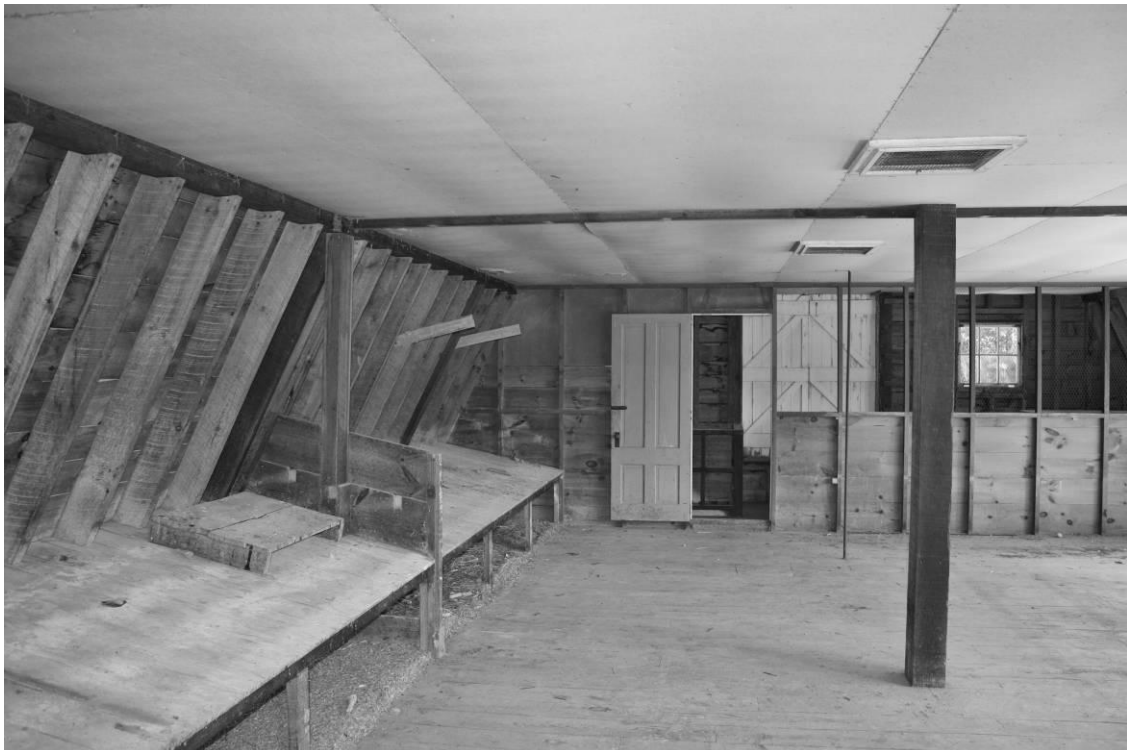
Photo # __15__ Description: Poultry barn, second floor interior (north building) Digital file name: NHA0010_15 Direction: north
