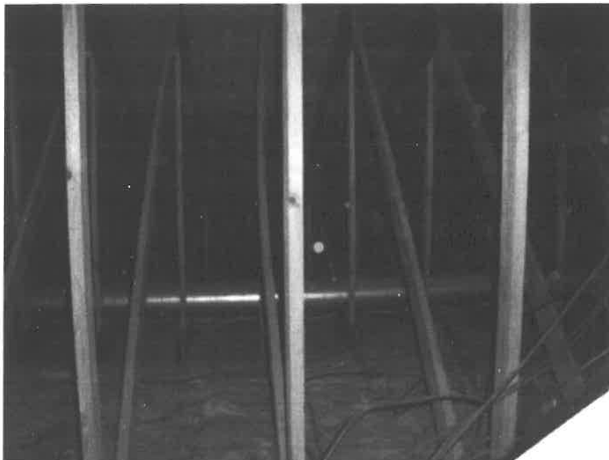
Photo 3: Bowed truss web diagonals, no thru-truss bracing.
