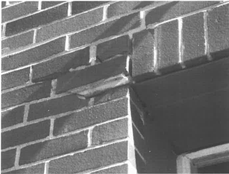
Photo 6: Damaged exterior masonry, west overhead door.
