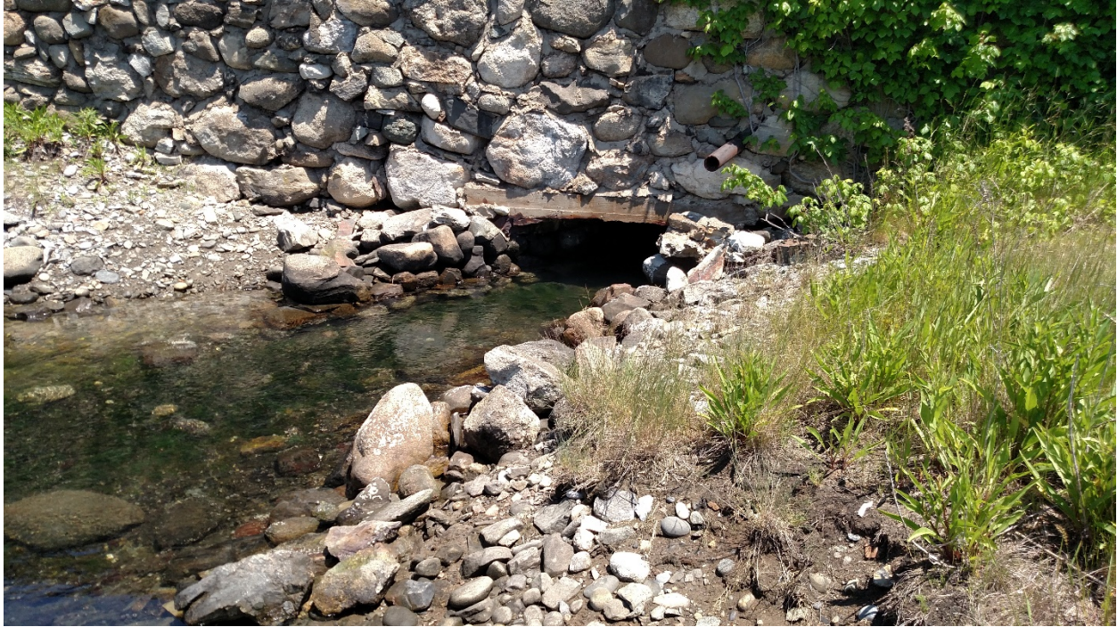
Photo 1: Philbrick's Pond Culvert (looking east) (7-2-2019) Stone weir at inlet to be removed and replaced with a precast concrete slab.
