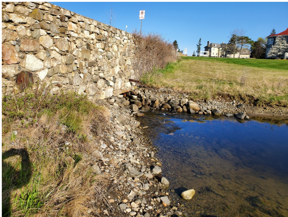
Photo 2: Philbrick's Pond Culvert (looking south) (5-7-2020) Riprap to be installed on slopes for inlet erosion protection.
