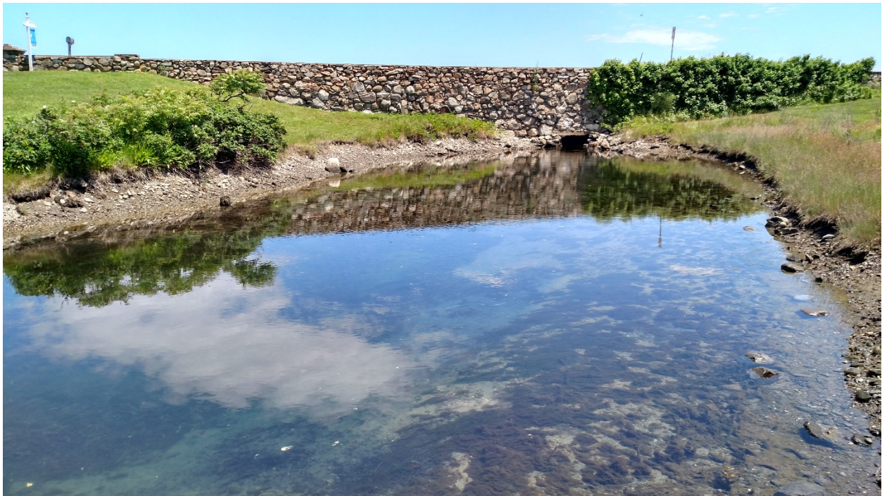
Photo 4: Philbrick's Pond Culvert (looking east) (7-2-2019) Stream channel to be regraded to improve stream flow.
