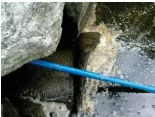
Figure 4 Chipped VC pipe, with voids over pipe
