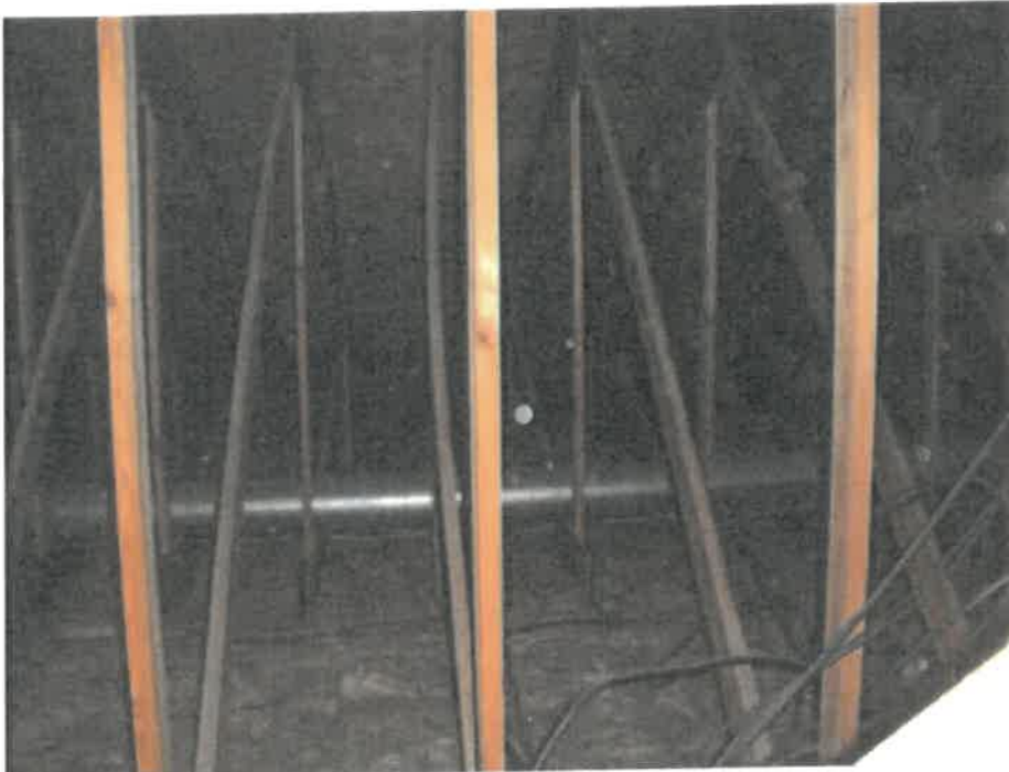
Photo 3: Bowed truss web diagonals, no thru-truss bracing.
