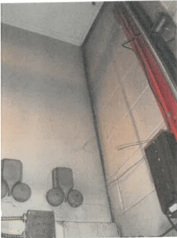
Photo 8: separation of south gable end wall (at right) from intersecting interior wall (left).
