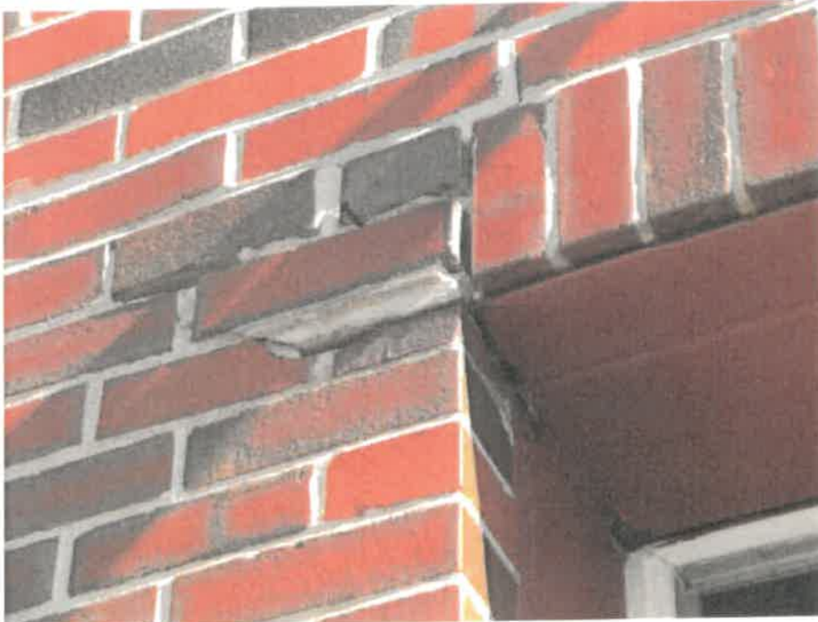
Photo 6: Damaged exterior masonry, west overhead door.
