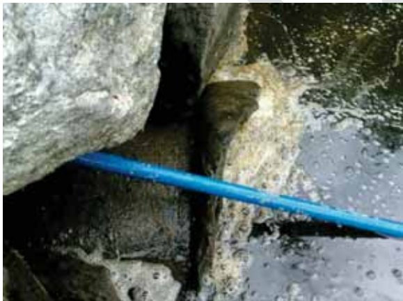
Figure 4 Chipped VC pipe, with voids over pipe
