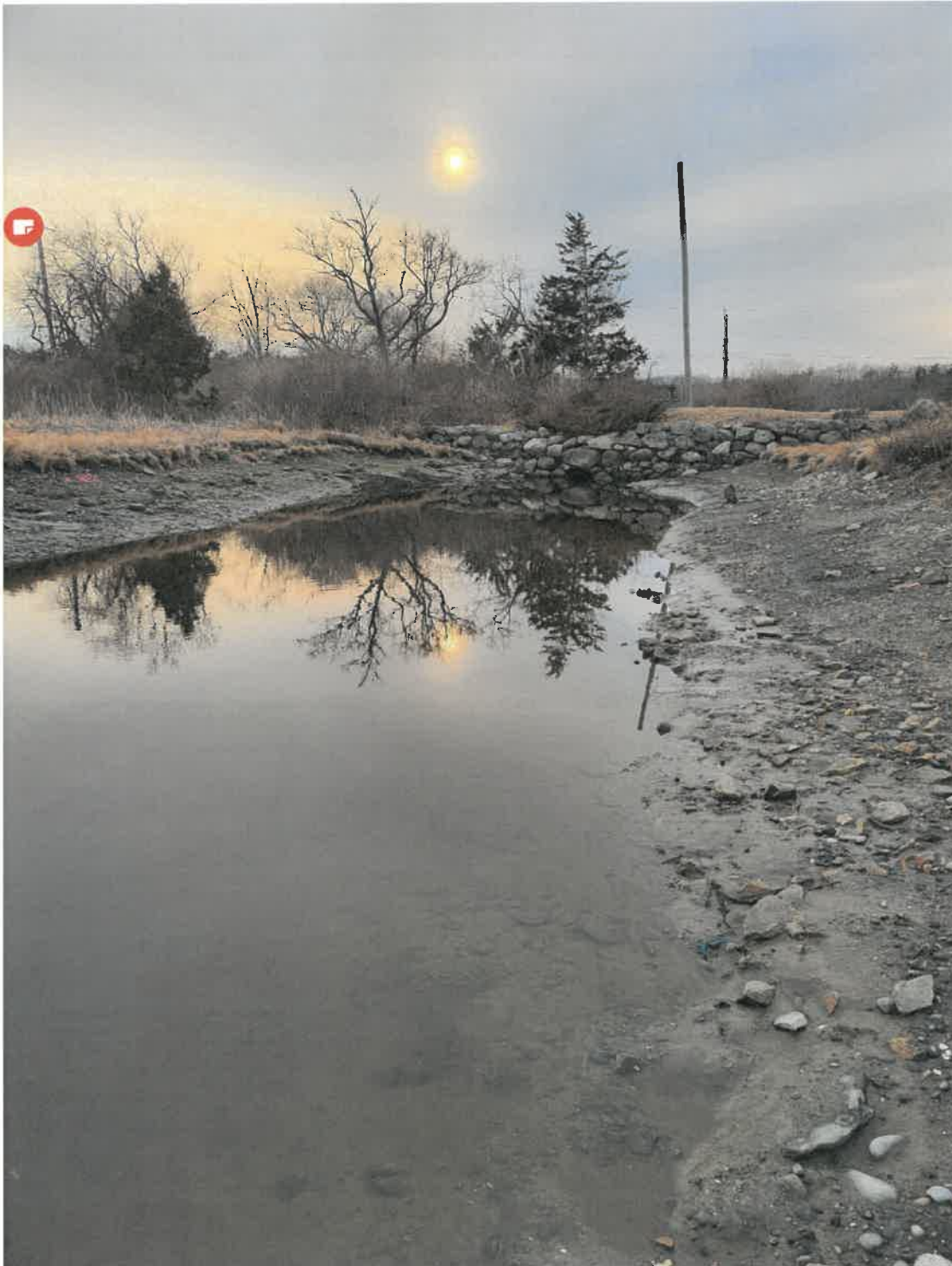
2. Philbrick Pond Trolley Berm, March 15, 2022
